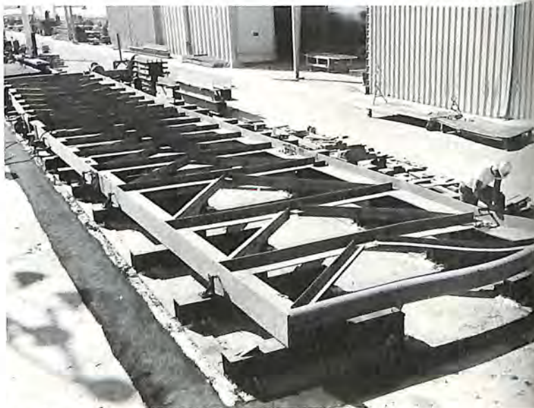
Tie truss for the deep space tracking antenna at Goldstone, Calif., is laid out at the Rohr Corp. plant.
