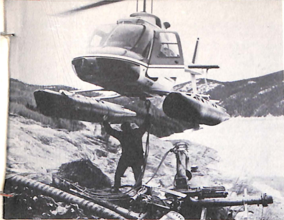
A Bell JetRanger helicopter, equipped with fixed floats, prepares to hook up a water cannon, used to clean loose rock from the side of a steep cliff. The helicopter relocated the equipment in two hours. It would have taken a full work crew two days to do the job.
