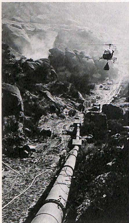
One of the well known Bell Model 47 helicopters that is helping in the construction of a water line to a California rocket site.
