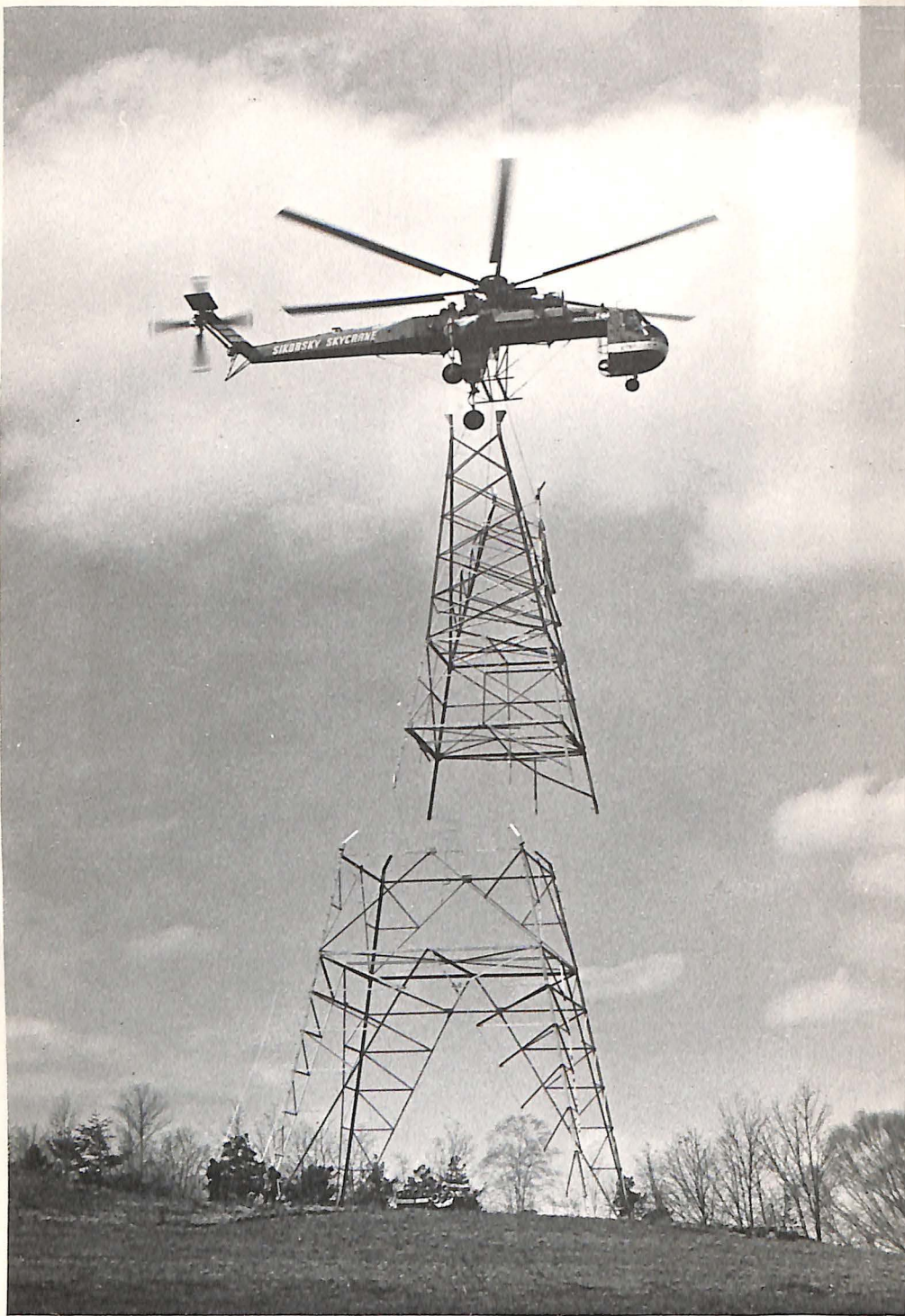
A Sikorsky S-64E Skycrane (R) helicopter places waist section of transmission tower on previously set foundation. In addition to erecting powerlines, helicopters are being used in heavy construction projects as well as in logging and ship-to-shore offloading of cargo.
