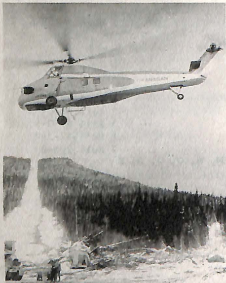
An Okanagan Sikorsky S-58T helicopter picks up a load of concrete during construction of a ski lift at Mt. Tom, Kamloops, British Columbia. Concrete is poured from the helicopter to form footings for ski lift towers.
