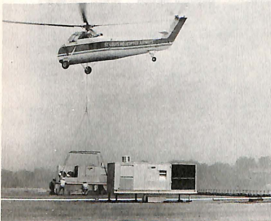
In Missouri, one of St. Louis Helicopters' Sikorsky S-58's on a cost-effective construction job.
