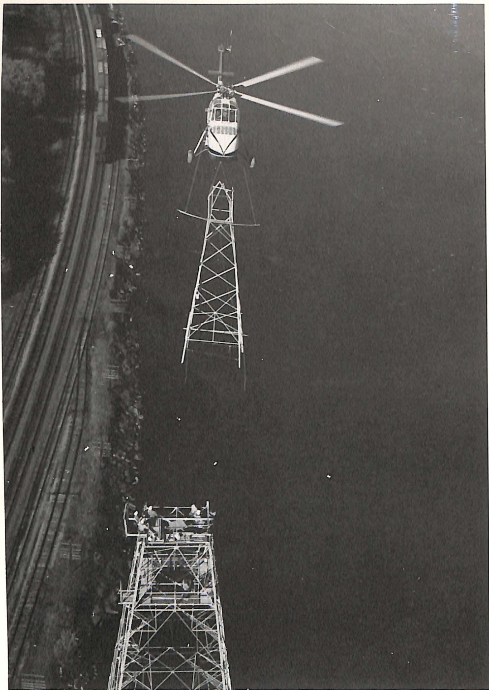
The Helicopter Construction Tool. Power-line transmission towers are erected across mountains, rivers and ravines by helicopter. Here a Sikorsky S-58 does another "impossible" job, as it flies the top tower section in a sling load for precision placement by the waiting crew.
