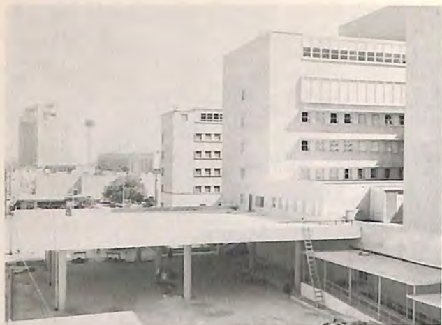
Nearing completion— the rooftop heliport at Baptist Memorial Hospital, San Antonio, Texas.
