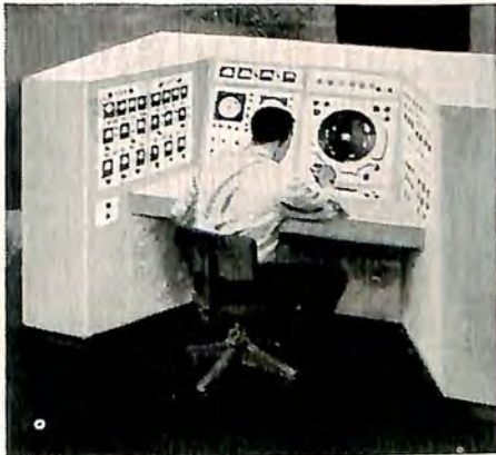
CENTER OF OPERATIONS for FPS-35 installation is MAJAC—Monitor, Anti-Jam and Control Console.
