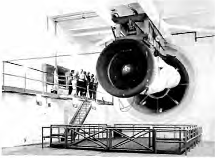
PAC Group's Pacific Airmotive Engine Division completed and put into operation a new test cell capable of accommodating engines up to 100,000 pounds thrust.
