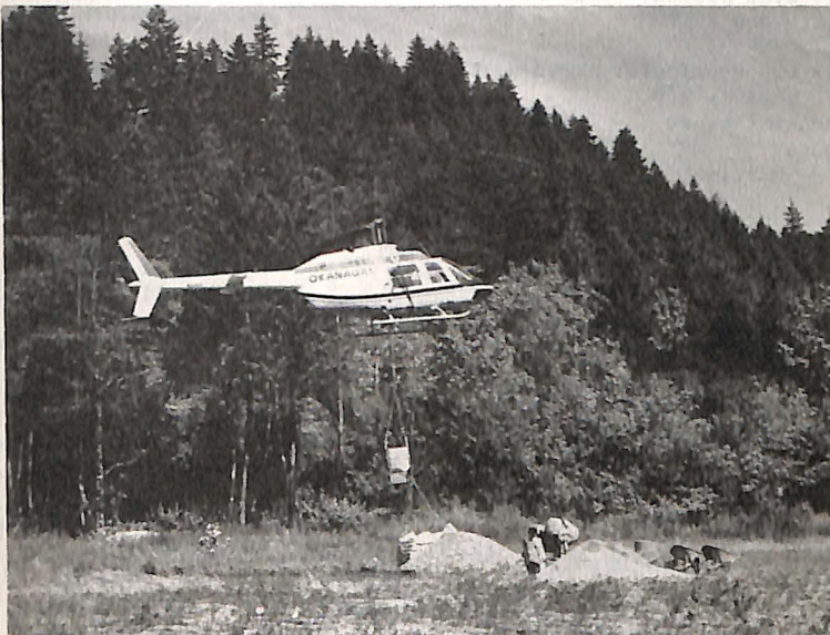
Okanagan Helicopters Ltd., JetRanger is shown working on the Peace River transmission line project in British Columbia. The turbine-powered Bell aircraft makes a sling-load pickup of construction materials for delivery to a tower site.
