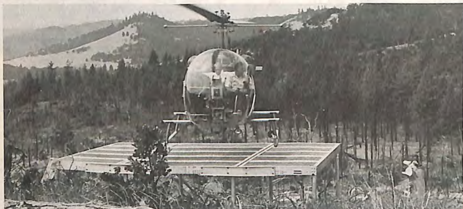
And now there is an "instant" heliport. This portable pad can be air-lifted to a temporary site by a light helicopter, thus providing a convenient landing area in a variety of types of terrain, from brushy slopes to swamps to tundra.
