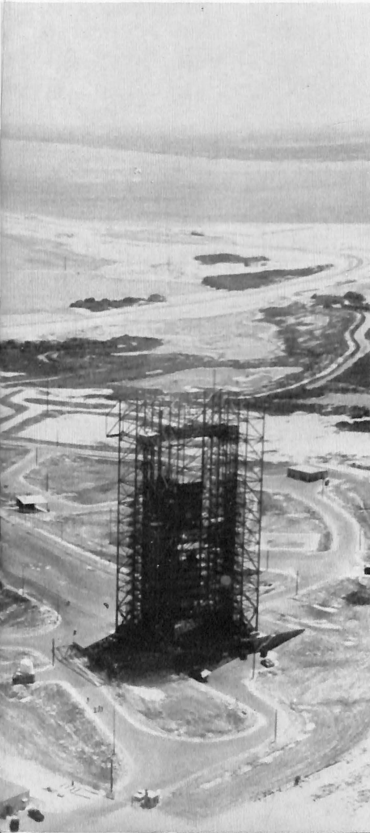
The launch facility for the Martin Company Titan III-C at Cape Kennedy, Florida, is designed for efficiency.
