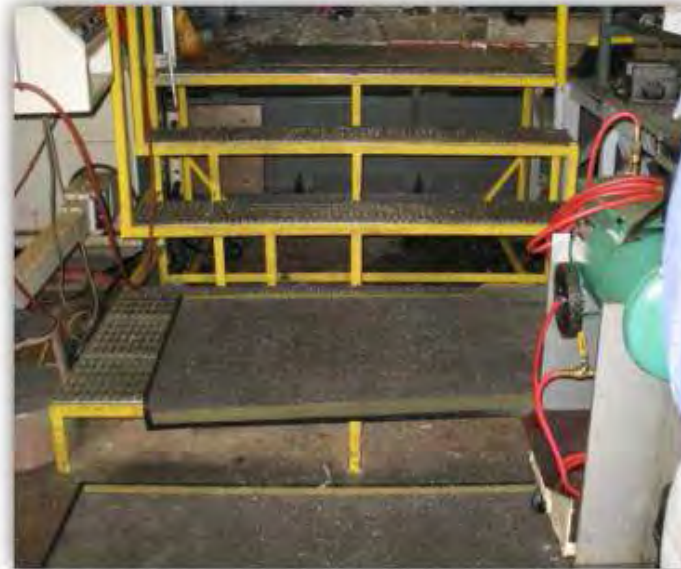
Loose mats on stair treads
