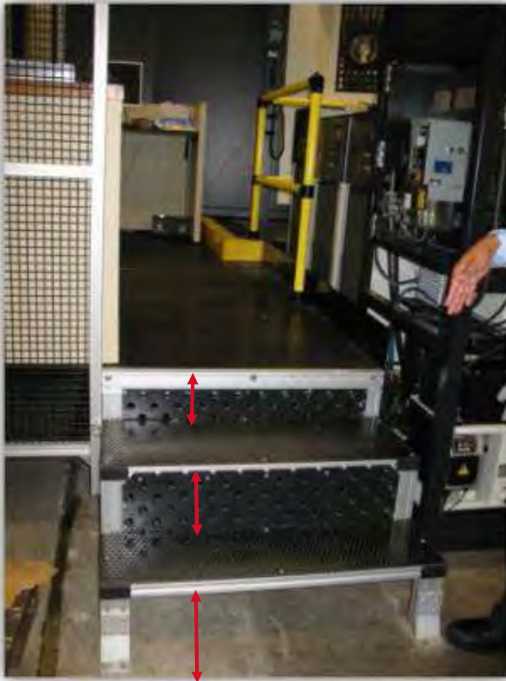
Equipment stair treads inconsistent in height and width. Limited visibility on a couple stairs.
