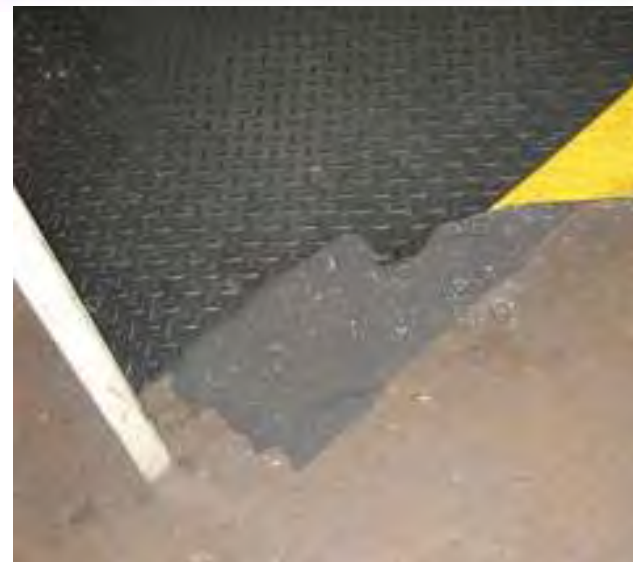
Worn mats may cause trip hazards
