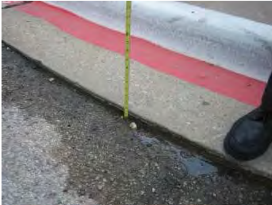
Transition Between Concrete and Asphalt (1" variance)
